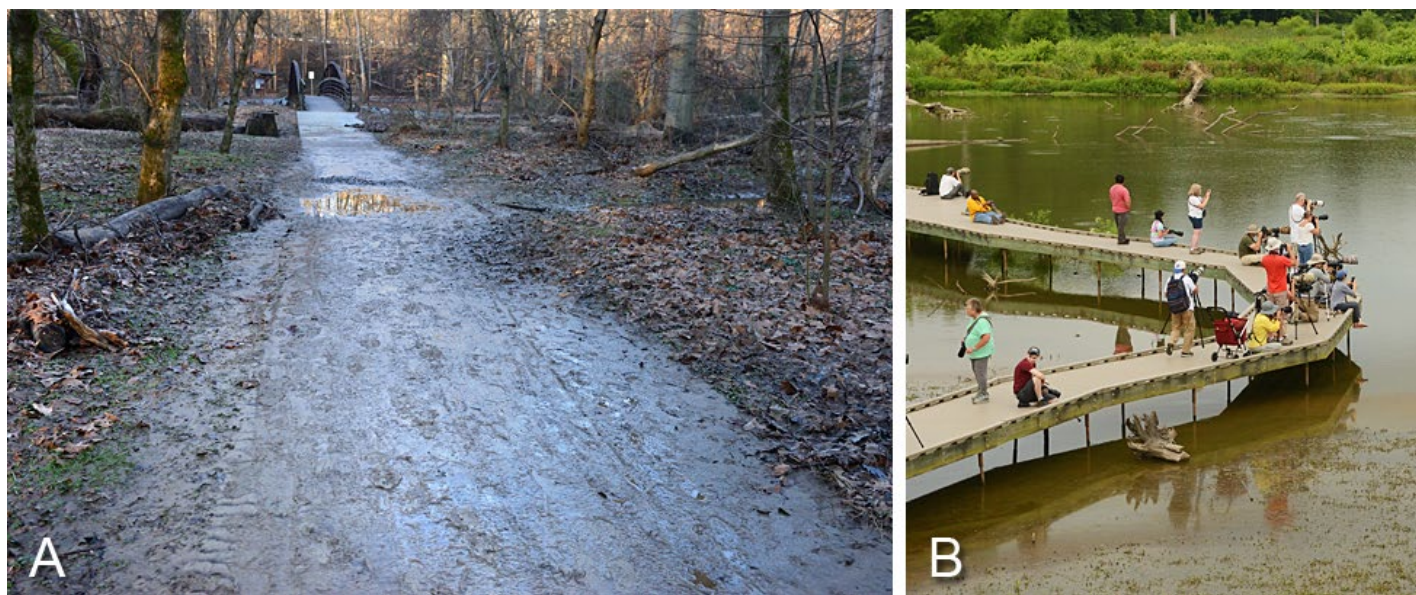
Figure 5. Pavement can often prolong a trail's maintenance even in poorly chosen locations. In the wrong place, a trail will flood regardless of what is on its surface. Pavement does not part water, leaving a puddled and mud-covered blacktop (A). Silty layers render pavement dicier than walking across a muddy field, discussed in the article, Slippery When Wet (December 2018). Mosses, algae, and other biofilms also make frequently wet trails slick. Furthermore, water can undercut and erode asphalt trails, which is what happened many years ago at the Shanes Creek trailhead by Roberts Road. Boardwalk trails (B) are the best way to access wetlands on foot. Replacing the half-mile boardwalk and two overlook platforms at Huntley Meadows Park in 2011 cost $600,000, which comes to around $178.00 per square foot for replacing wooden planks with recycled plastic ones—there were no structural additions that would further inflate the cost. This price tag is prohibitively
