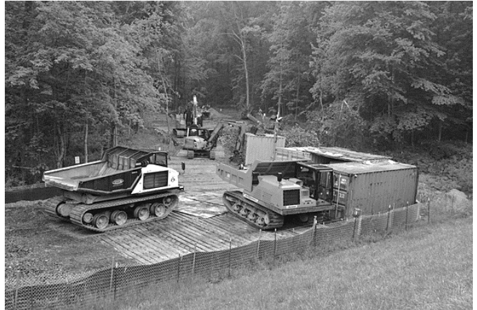
The construction entrance at Roberts Road has a staging area (foreground). Wood planks protect the soil from earthmovers traveling along the work zone.
