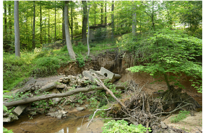
Figure 1. This “before” image reveals the destroyed storm drain outfall and massive erosion next to private property.
