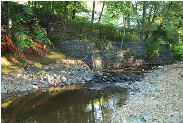
Figure 8. The restoration’s upstream terminus (left) used modern approaches to replicate a natural creek. It is a more conducive environment for aquatic life than the gabion walls (center) to control bank erosion, which were installed decades earlier. This wall and the concrete-lined portions of creek bed with “speed bumps” (not seen here) are outdated waterway control methods.
