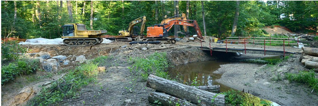
Figure 3. A temporary bridge enabled earthmovers to cross Rabbit Branch and perform work upstream. Boulders on the left await placement in repairing the water’s course from a storm drain outfall. Logs from fallen trees (center) will integrate into the stream bank and provide favorable habitat for aquatic life.
