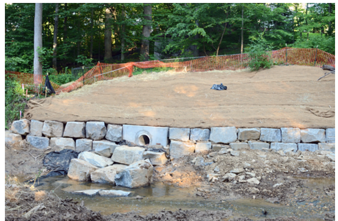
Figure 2. The “after” shot of the restored area shows a new outfall where stormwater hits stone boulders. A rock wall protects the hill from churning floodwaters. Until native restoration plants arrive, coir and straw promote grass growth that retains the soil. The county and other institutions are getting away from synthetic lawn netting since it inevitably becomes another source of plastic waste polluting the environment.
