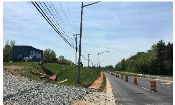
Sidewalks going in while looking southwest along Guinea Road from the Bronte Road intersection
